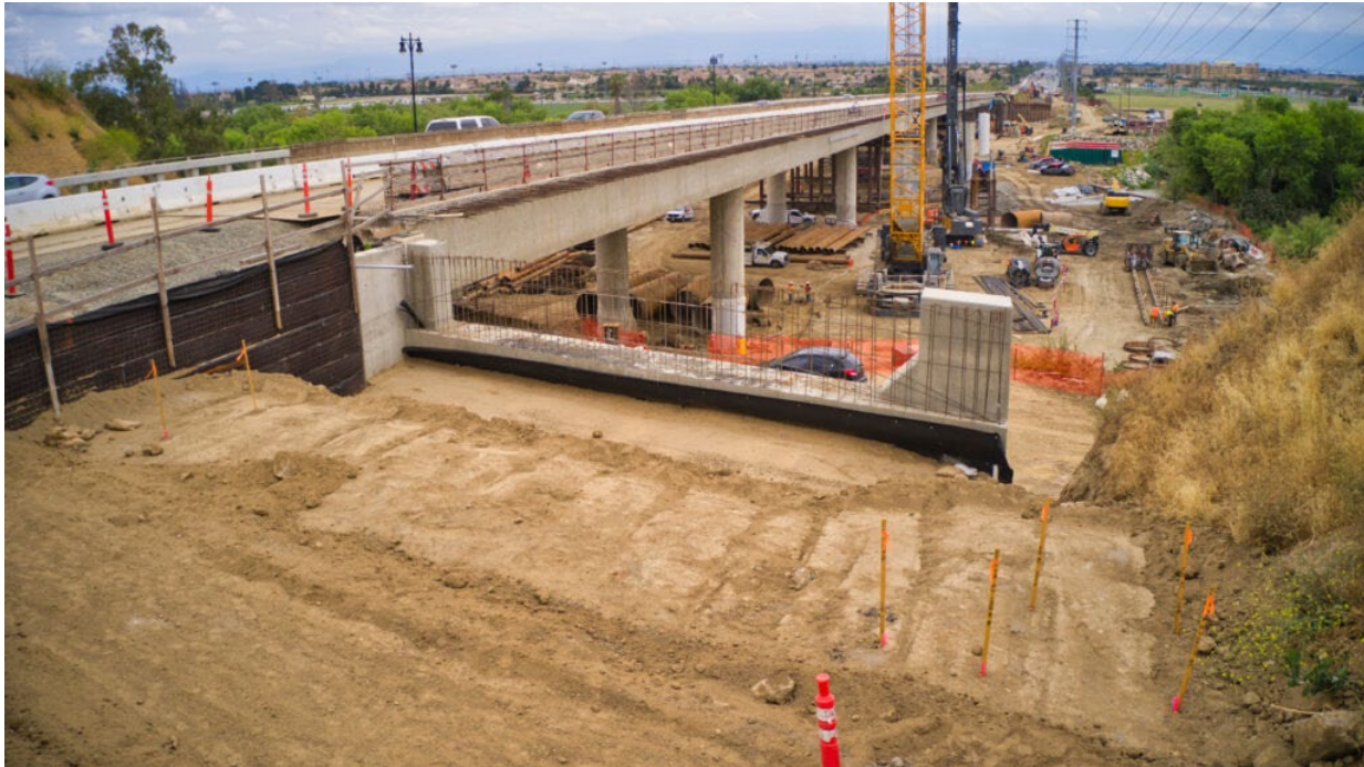
Construction progress on the Hamner Ave Bridge Project. Image Source: City of Norco.
