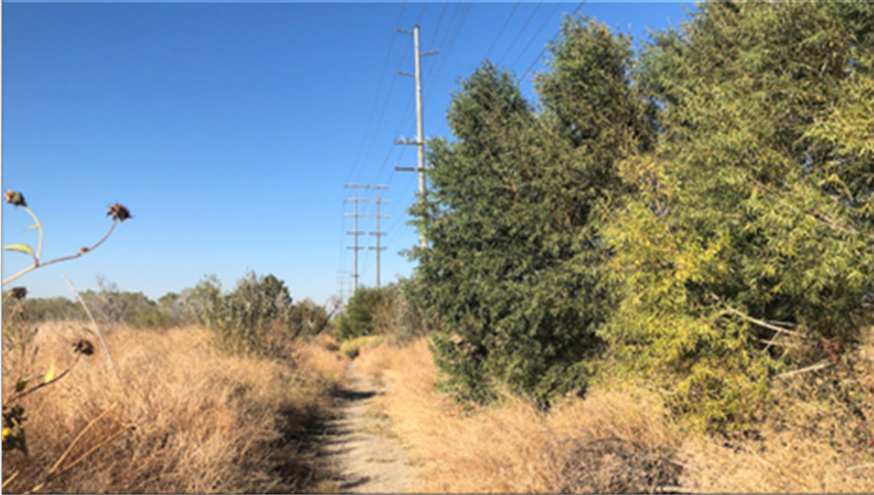
November 4, 2023: Towers and lines surrounded by growth and a nearly impassable service road.
